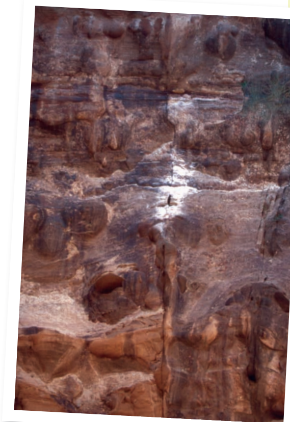
▲ THE BOTTOM OF THE ROUTE SHOWING ROCK SCAR FROM WHERE THE ROCK FELL
